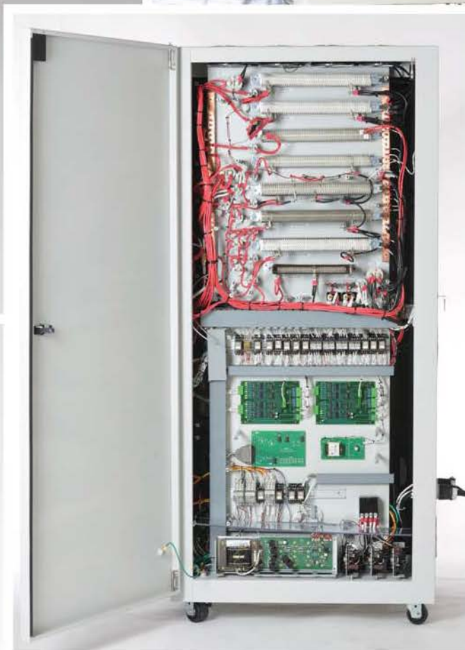
Side View with Side Door Open showing Bus Bars, Control Relays, Resistive Loads Communications and Relay De-Bounce Cards easy access for service and maintenance
