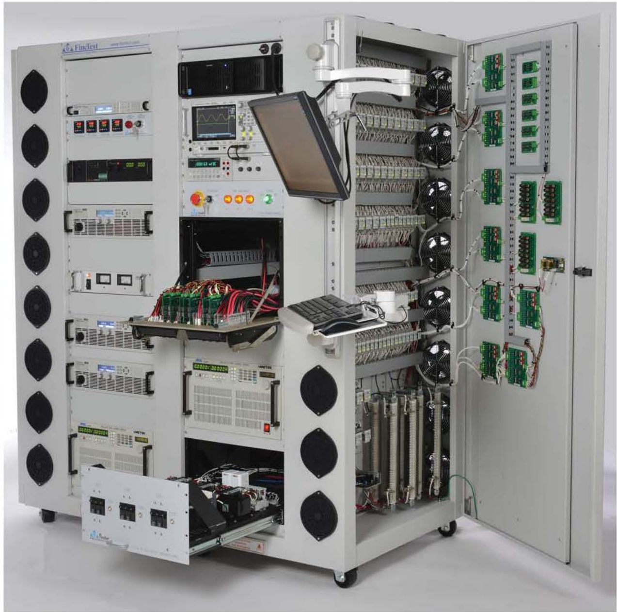
View of right-side door open showing Load Mux and Control Relays
