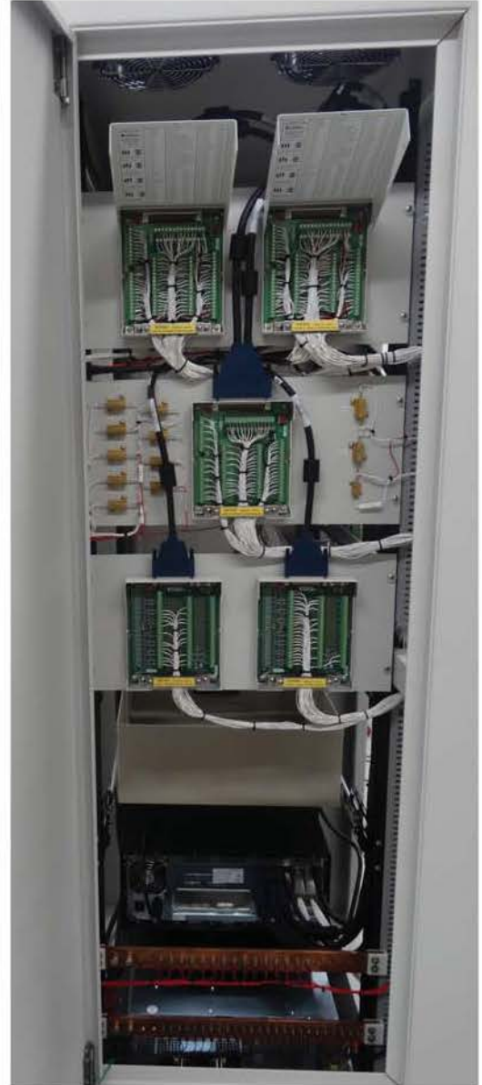
Rear View showing clean wiring
