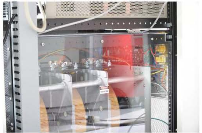
3 Phase 400 Hz Motor Driven Transformer
