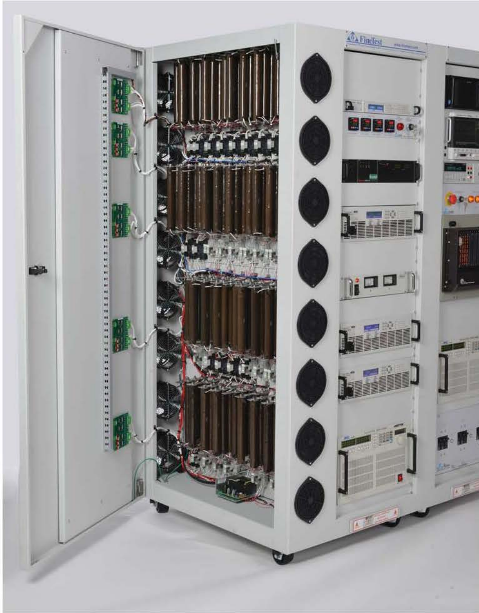
View of left-side door open showing Resistive Load Banks
