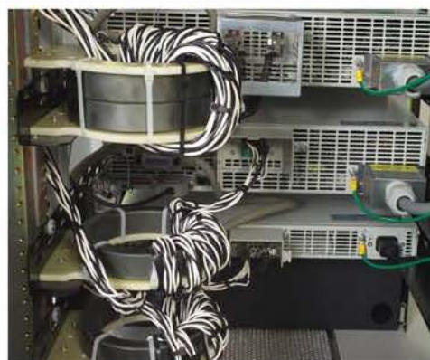
All Cabling through Ferrite Cores to minimize noise
