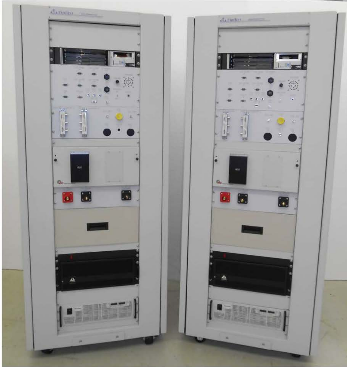
Front view of Simulator IO Racks #1 and #2
