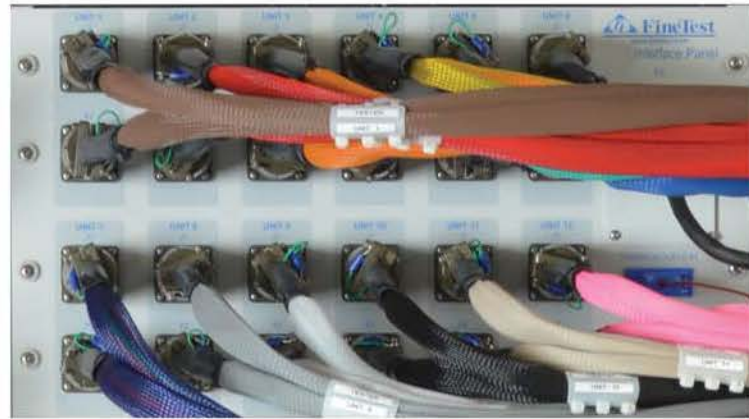
Rear System Interface Panel Close-Up showing 12 Unit Connections for Test Cables from Chamber to System
